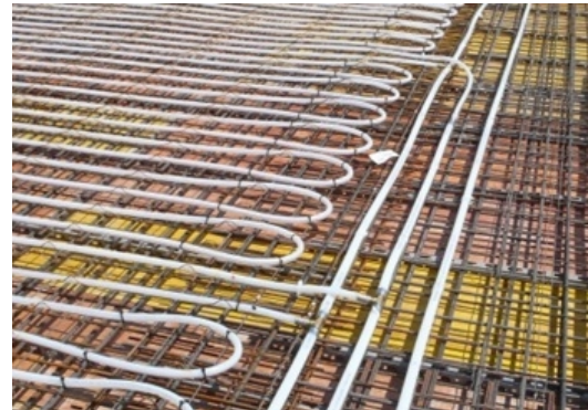
Thermally active slabs
