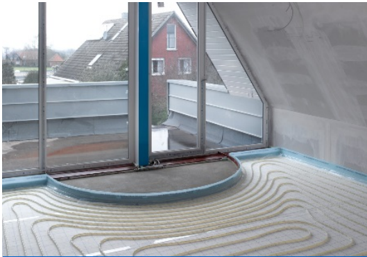
Radiant heating and cooling
