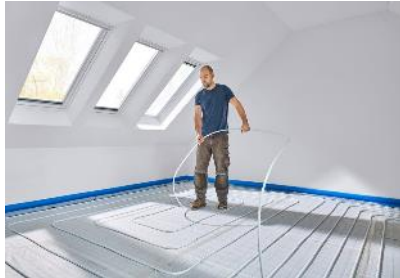
Radiant heating and cooling
