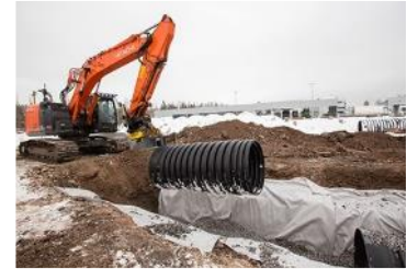
A cost-effective and reliable stormwater solution Volvo's Warehouse, Vantaa, Finland
