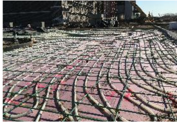
Scheels department store saves energy costs with radiant heating and improves safety with snow/ice melting Minnesota, USA
