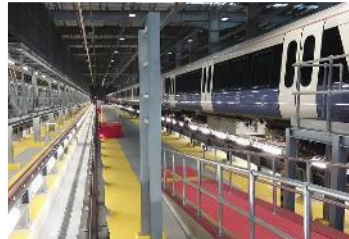
Uponor TABS offering safe and comfortable temperatures for train maintenance teams in one of the largest rail depots in Europe: London, UK
