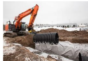
A cost-effective and reliable stormwater solution Volvo's Warehouse, Vantaa, Finland
