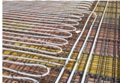
Thermally active slabs
