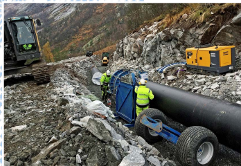
Water supply in demanding terrain: Glomfjord, Norway
