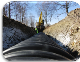
First installation of large-bore Uponor IQ pipe in Örebro, Sweden, featuring a unique inline extrusion of the socket
