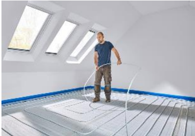
Radiant heating and cooling
