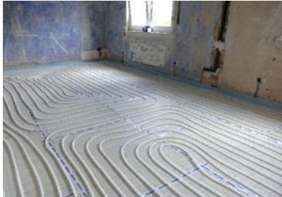
Radiant heating and cooling
