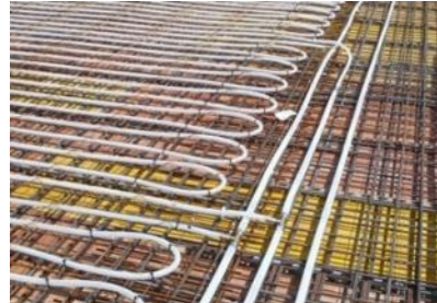
Thermally active slabs
