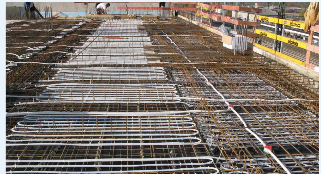
Thermally active building systems are built into the concrete ceiling. Prefabricated pipe modules are suspended from the upper reinforcement of the concrete ceiling and then encased in concrete.
