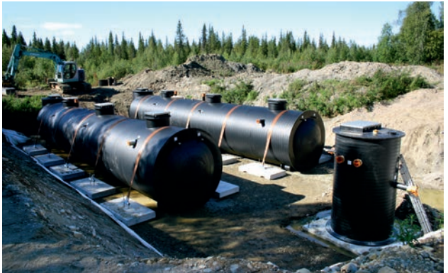
Kitilä, Finland: The WehoPuts 400 wastewater treatment plant built for the Kaukonen village was found the most rational solution when compared with transporting sewage or building a pumped transmission pipeline several tens of kilometres long. The treatment sludge can be composted on the treatment plant premises.
