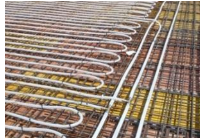
Thermally active slabs
