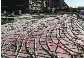
Scheels department store saves energy costs with radiant heating and improves safety with snow/ice melting Minnesota, USA
