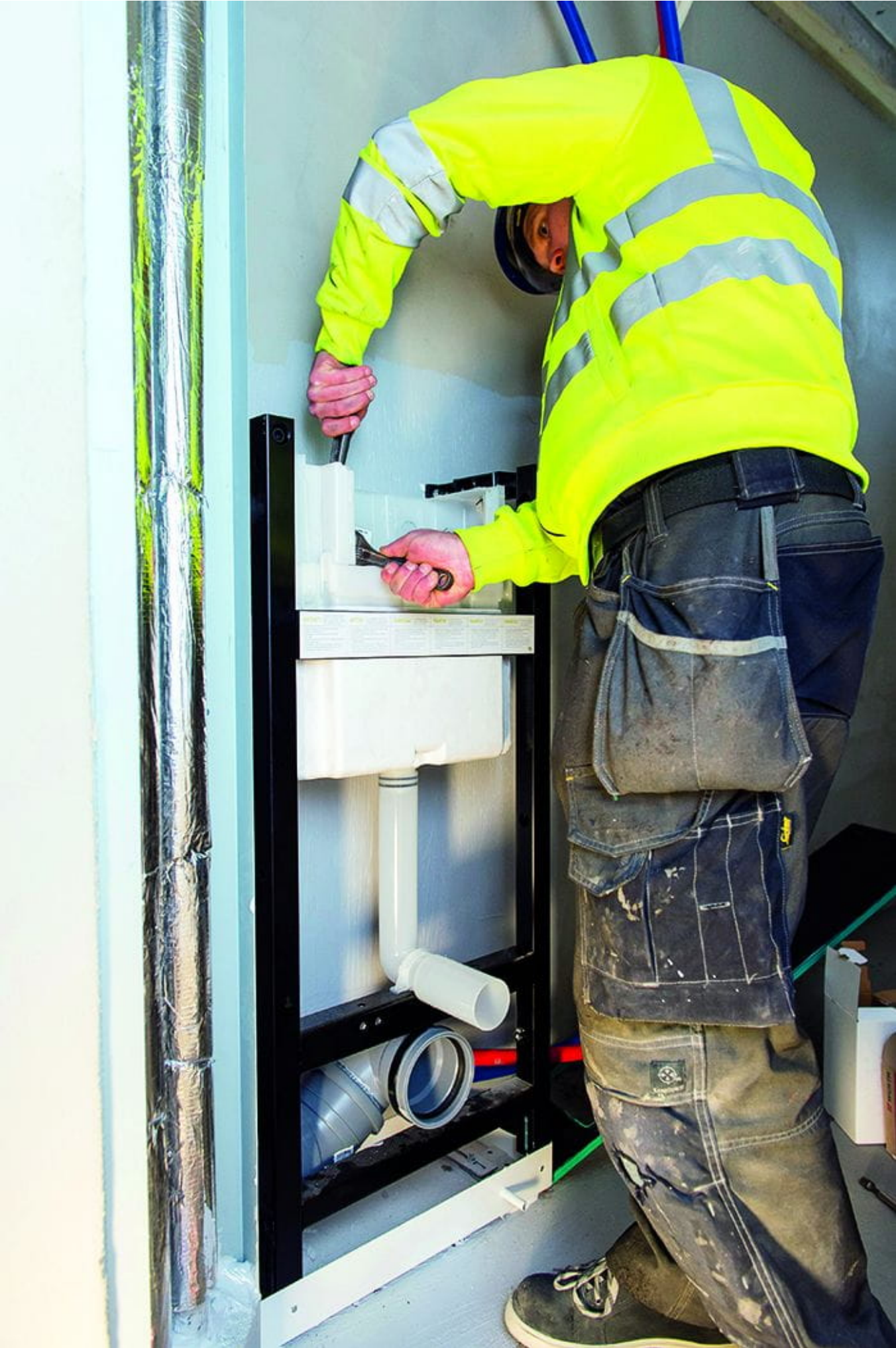
A housing company in Turku saved time and money using Uponor's Cefo pipe overhaul
